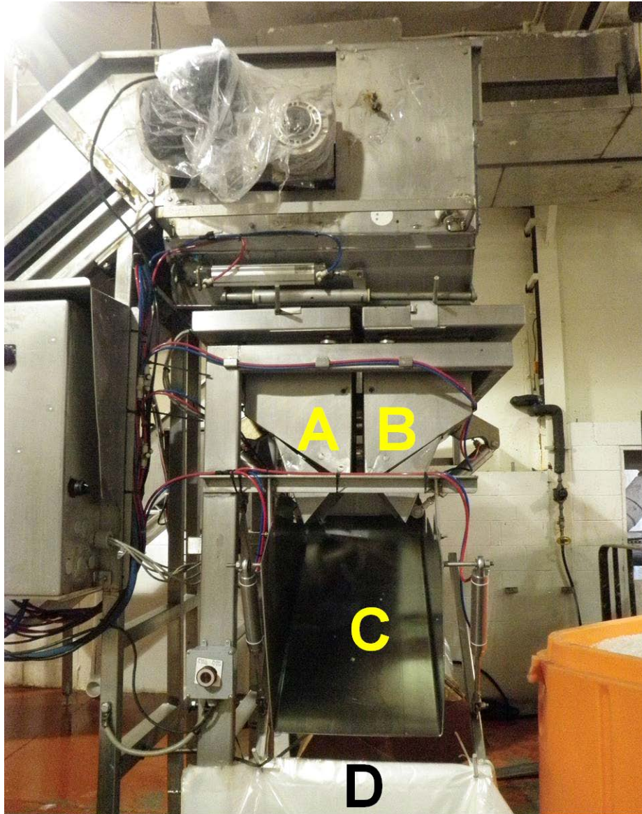
Figure 29. Each of the two hoppers pictured here (A and B) has an electronic scale to verify the total weight of the fish. As one hopper opens to drop the fish down the chute (C) and into the packaging (D), the other hopper is being filled and the contents weighed and later opens as the first hopper begins to fill again.
