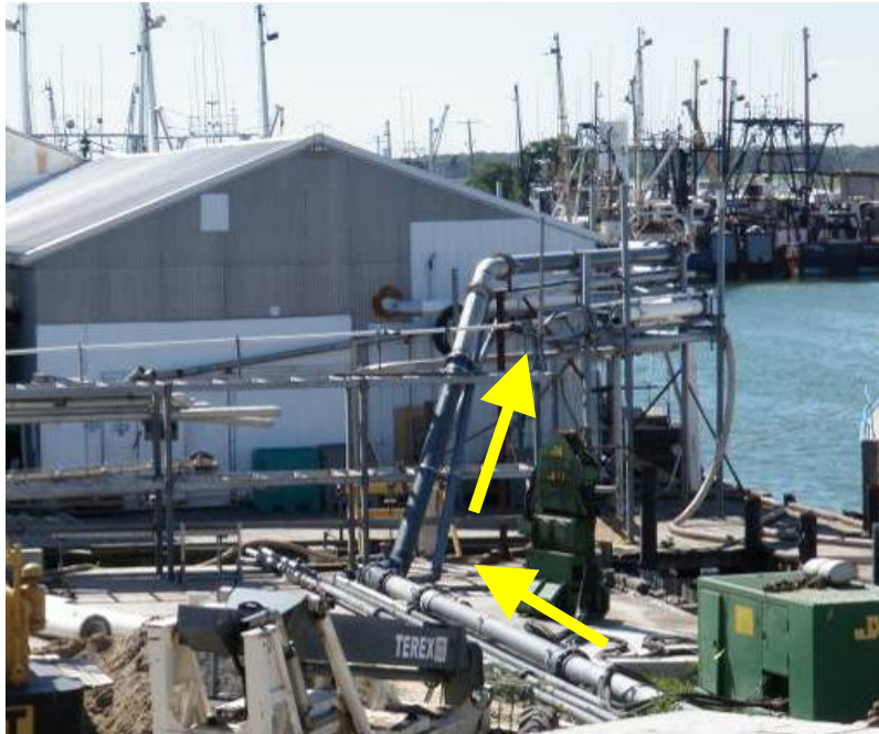
Figure 24. Transportation pipes and hoses entering the processing facility after coming from the dock.
